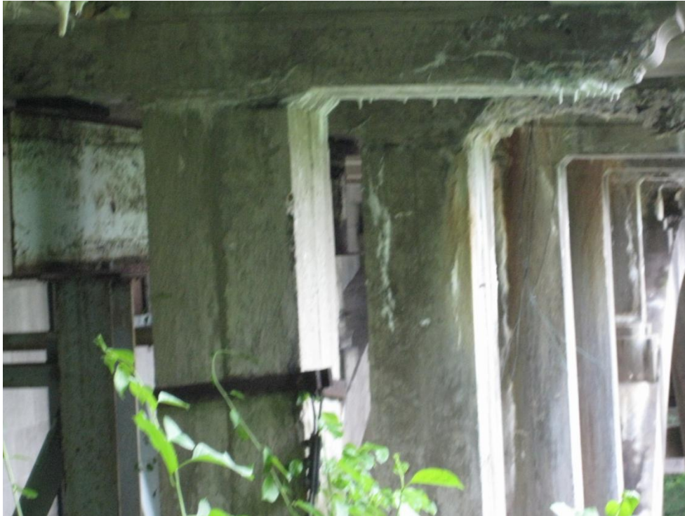
Figure 4.7c –Lack of cracking between the spandrel columns and the deck (photograph taken in June 2009).
